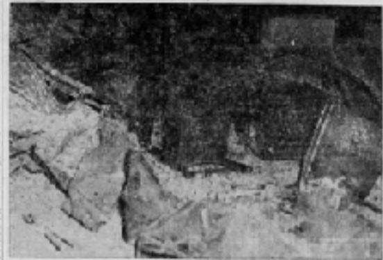
This close up was taken to show the destruction of the building that caused the destruction of Section School. Students will have to use their private tables and chairs. The building is being repaired. (Left photo)
